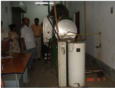
Unused Autoclave in a primary health centre in Maldah
